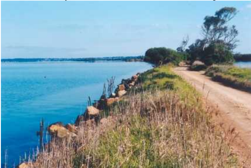
Silt jetty with no natural erosion protection.
